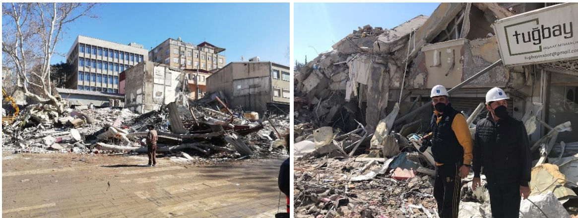
Figure 5.1. Building Collapse in Antakya and Kahramanmaraş
