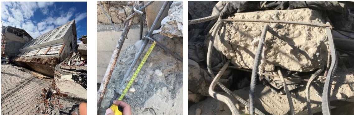
Figure 5.3. Overturning due to soil liquefaction and insufficient joint reinforcement detailing
