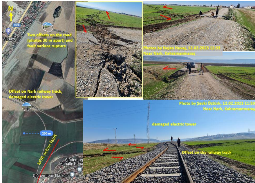
Figure 8.4. Surface rupture, offset, cracks and damages on railway tracks and roads, as well as a damaged electric tower, near the surface rupture (Narlı, Kahramanmaraş). (Active fault data is taken from Emre et al. (2013)).
