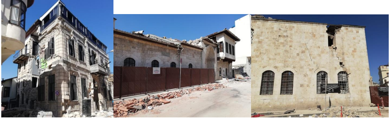
Figure 5.9. Damage in masonry structures
