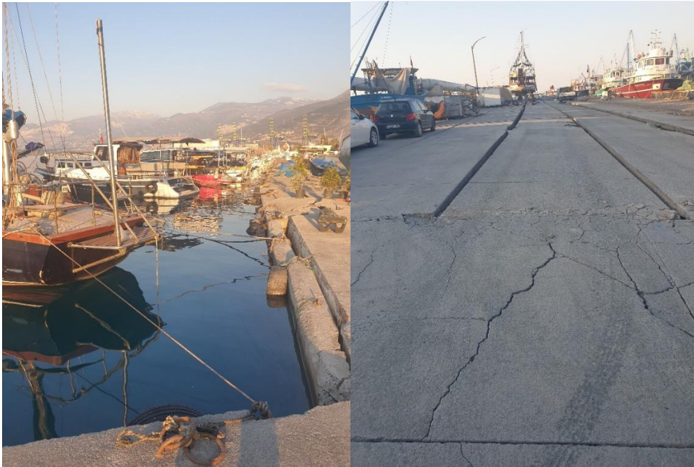
Figure 7.4 Structural damage at İskenderun Fishery Port
