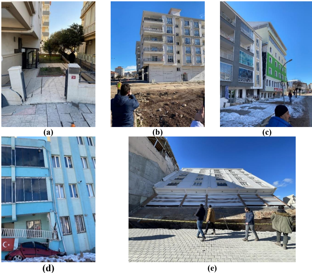
Figure 4.4. Poor foundation performance in a) Çay District / İskenderun / Hatay ( 36.5911^{\circ}N , 36.1790^{\circ}E ), b) Hüriyet District / Gölbaşı / Adıyaman ( 37.778^{\circ}N 37.628^{\circ}E ), c) Yavuz Selim District / Gölbaşı / Adıyaman ( 37.788^{\circ}N , 37.642^{\circ}E ), d) Yavuz Selim District / Gölbaşı / Adıyaman ( 37.788^{\circ}N , 37.642^{\circ}E ), e) Yavuz Selim District / Gölbaşı / Adıyaman ( 37.78827^{\circ}N 37.64879^{\circ}E )
