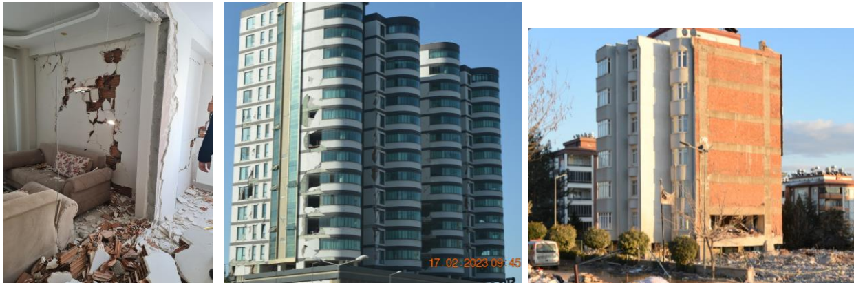
Figure 5.8. Infill wall damage examples
