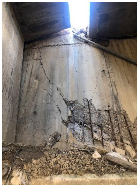
Figure 6.7. Abutment wall concrete spalling
