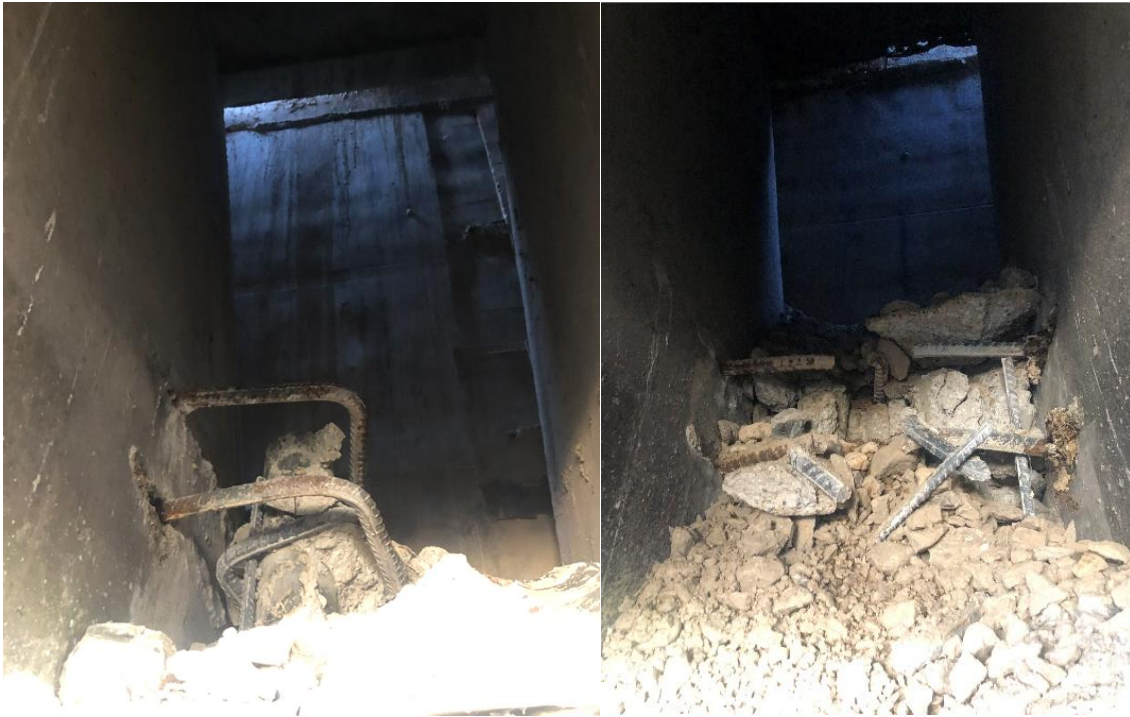
Figure 6.6. Shear key damage
