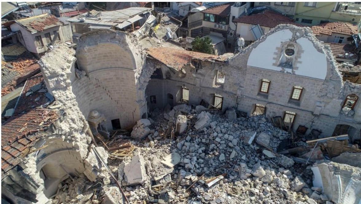
Figure 9.7 The Antakya Rum Orthodox Church after the earthquake 5
