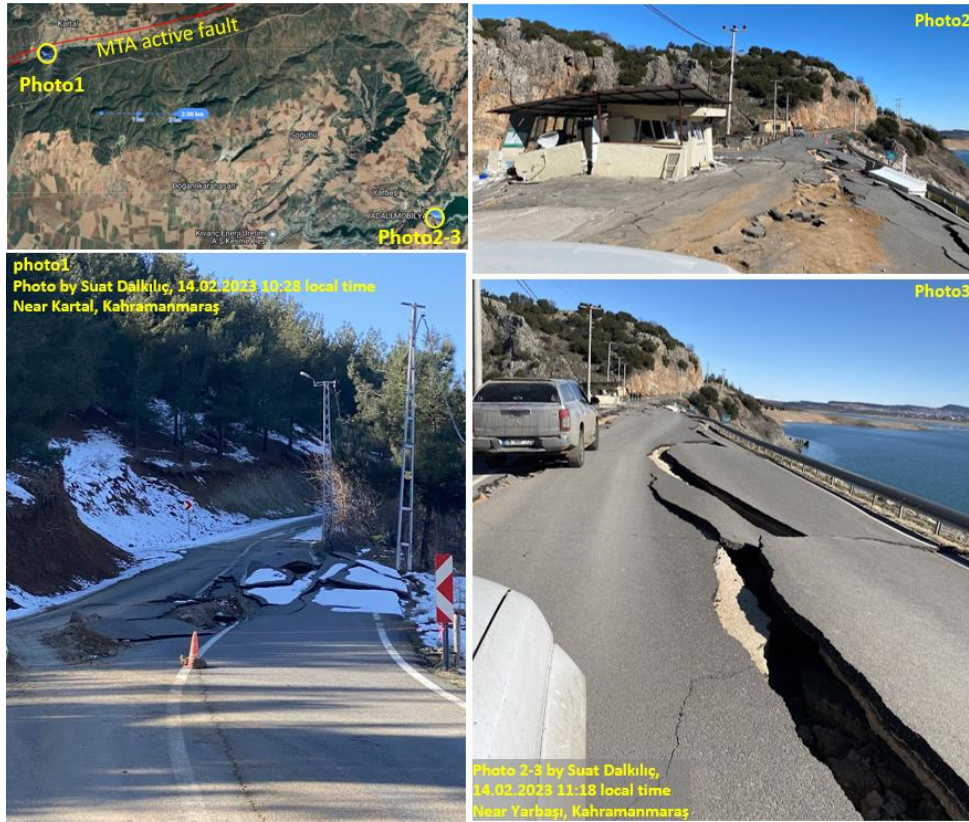
Figure 8.8. Landslides and surface cracks on the roads, near Kartal and Yarbaşı, Kahramanmaraş (Active fault data from Emre et al. (2013)).
