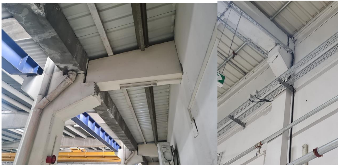
Figure 5.7. Corbel damages in Gaziantep
