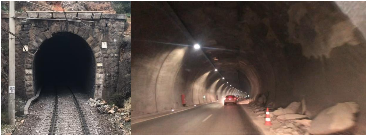
Figure 6.9. Tunnel portal movement and concrete spalling
